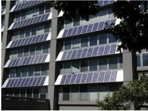
Fig. 14: PV shade Screens (Finland)
